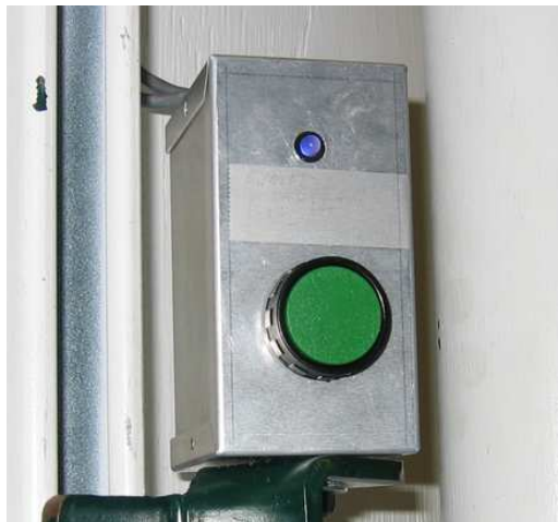
Figure 2: Motor reset button, located in the hutch near the door
