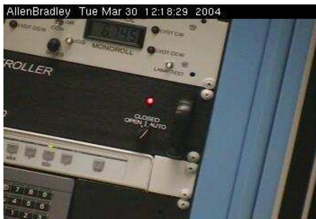
Figure 41: Shutter controller showing open shutter status
